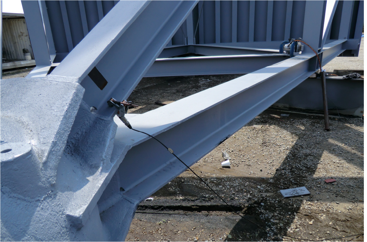
Figure 5: View from hinge point of gate, showing vibrator location of the right, and accelerometer on the left.
